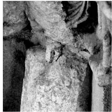
Top of one of the colonnettes fixed with metal pin
