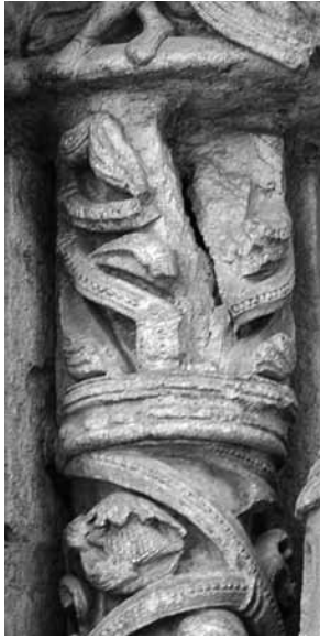
2 - nL1t probably from a Xavier shaft carved in group 2, and like '1' placed by G. Looks like it was placed upside-down with the end-ring at the base. It is split where the metal anchor was drilled. It is 20cm high, which is the extra added to the door heights in that campaign.
